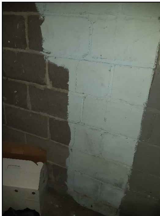
47. Typical minor cracks
