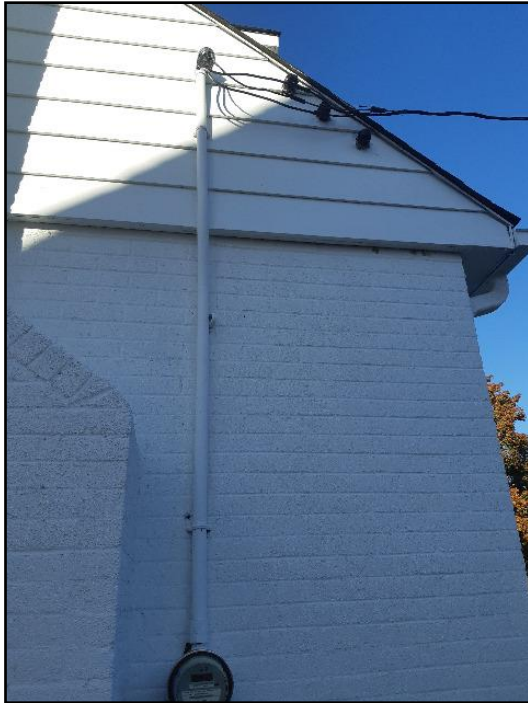
48. Overhead - cable type not determined
