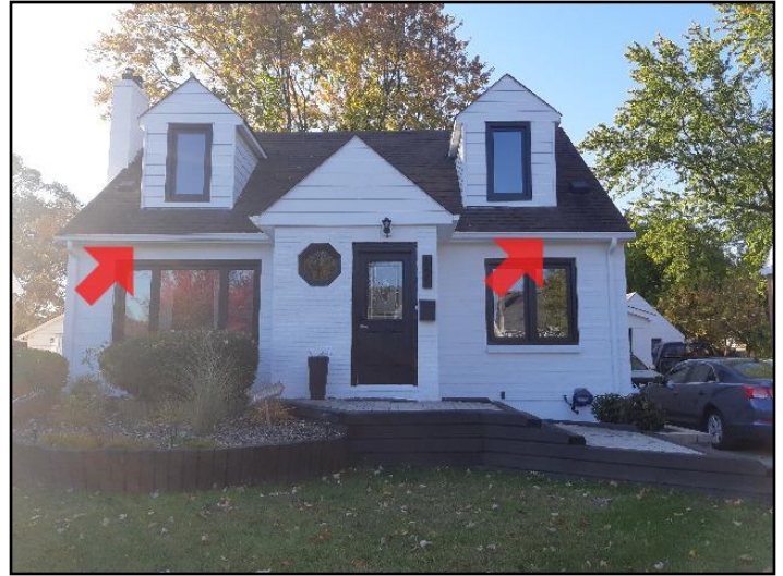
34. solid soffits lack of venting
