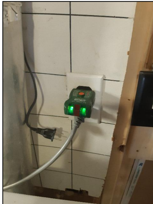
68. No GFCI/GFI (Ground Fault Circuit...
