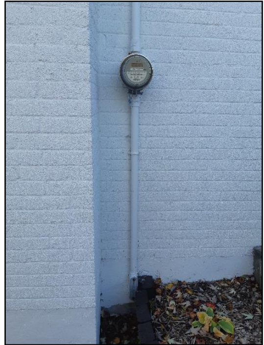
49. Overhead - cable type not determined
